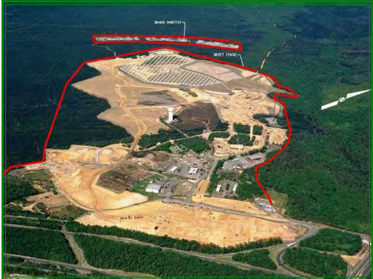
Figure 2. A 2007 aerial photograph showing a western view of the study site and the early stages of the commercial construction on the eastern and central portions of the site. The licensed landfill is centered on the western portion of the SPR property (highlighted with white lines), and retention basin D is located in the extreme western portion of the site (highlighted in white). The three Pine Snake mitigation and management fields are due west from the edge of the site (outlined in red lines). The perimeter exclusion drift fence and trap line is also outlined with red lines which surrounded the SPR property. Source: Walters, Inc.
